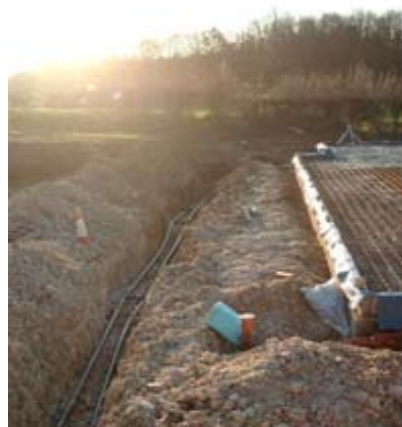
The Ground source heat piping at Petham Village hall
