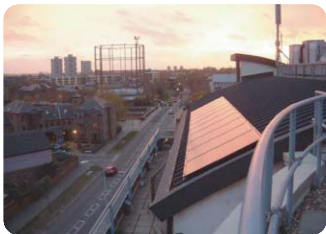
Youth Hostel Association, Rotherhithe. An installation carried out through the REAL initiative
